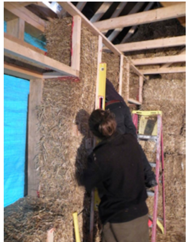
With Racusin and New Frameworks' hybrid straw-bale approach, the bales can be installed before the dense-pack cellulose is blown into the walls, as seen here, or after, as seen in the photo at the top of the article.
