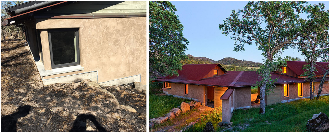
fig.1. Norrbom Road Strawbale Home - fires burned to the foundation on but not up the walls.
