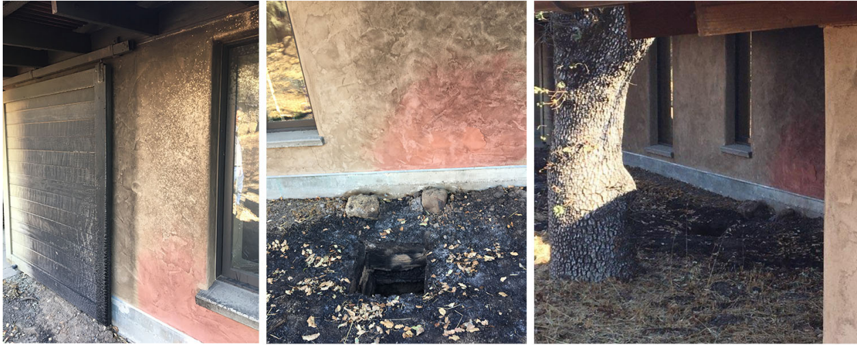
fig. 2. Norrbom Road - Mineral oxides in Natural Hydraulic Lime turn pink when heated.
