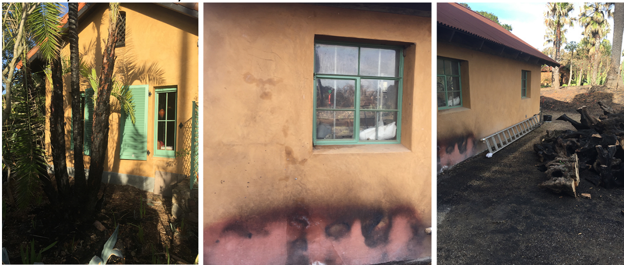
fig.3. Strawbale home on Lovall Valley Loop Road withstood fire against its walls.
