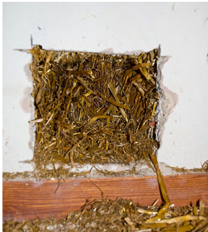
Fig.93 Bottom of damp wall at the Totnes House
