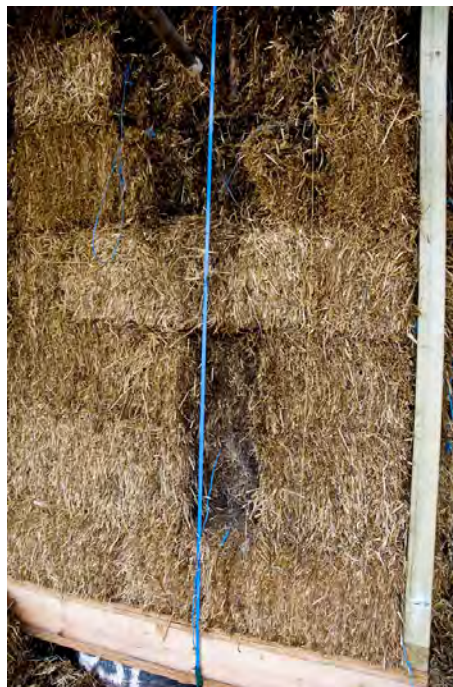
Fig.84 Water damaged straw has been removed from wall of Occombe Farm
