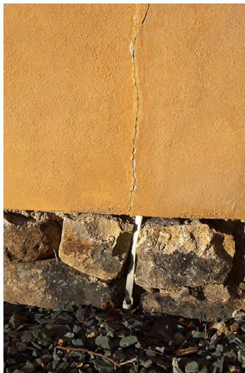
Fig.A20 Cracking in walls at Ecology Building Society
