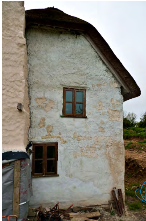
Fig.88 Poor quality of render on NE wall at Cuckoo Farm
