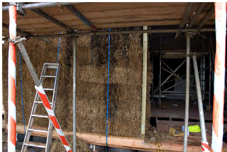
Fig.A39 Water damage to walls at Occombe Farm
