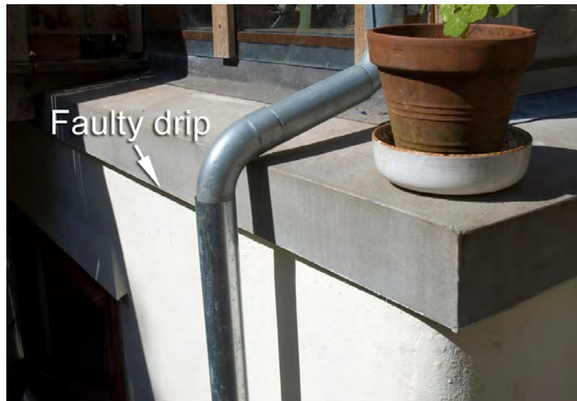
Fig.71 Location of faulty drip detail above bedroom 1
