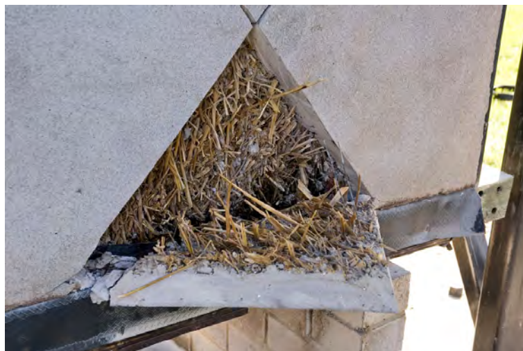
Fig.A11 Section of render removed from panel
