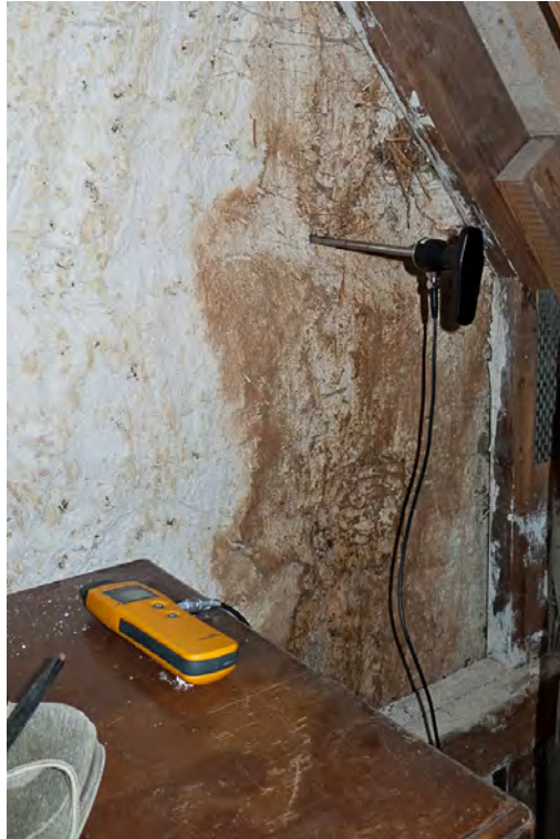
Fig.A36 Moisture damage to bedroom wall at Cuckoo Farm
