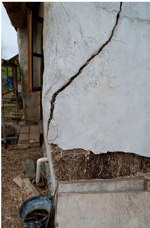
Fig.A35 Render falling off wall at Cuckoo Farm
