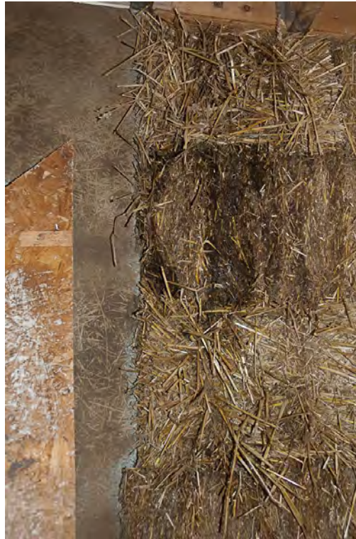
Fig.A23 Water damage at Atkinson Cottage
