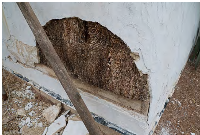
Fig.97 Corner of a wall at Cuckoo farm, where the render has failed.
