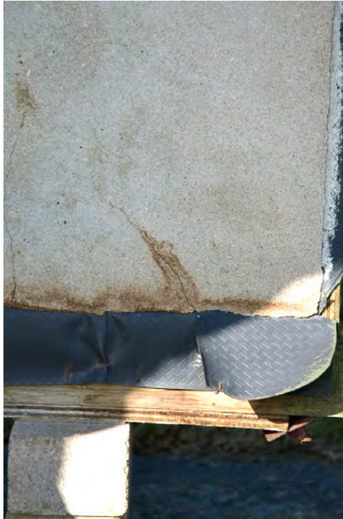
Fig.A10 Base of panel at UWE
