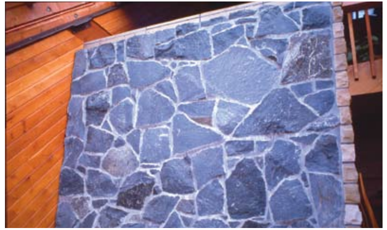
Fig. 2 A feature stone wall facing a north facing glass house is used in this house as the thermal mass
