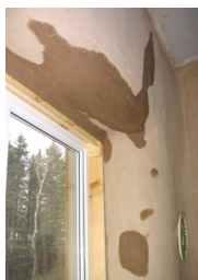
Wet walls from roof leaks (215)
