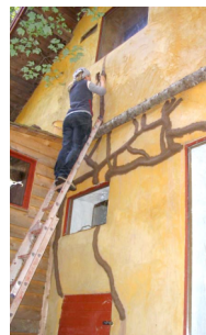
Cracks in earth plaster caulked with cob.
