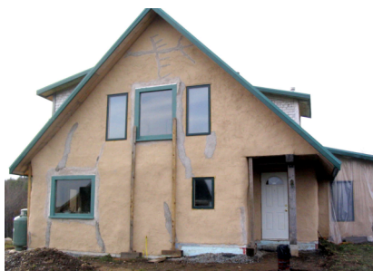
Cracks in cement plaster caulked with silicone.
