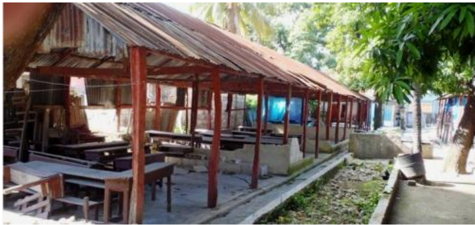
One of two classroom pavilions at the Interim Campus of The Center, prior to renovations.
