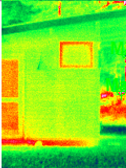
Figure 7a: Infrared Image bathroom no air leakage just bridging from foundation.
