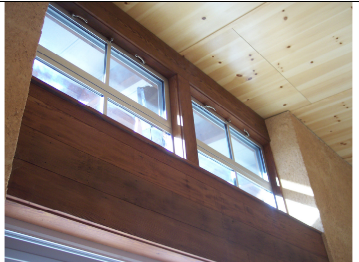
Figure 29: Very minor infiltration of fog in bottom right corner of right window during house depressurization.
